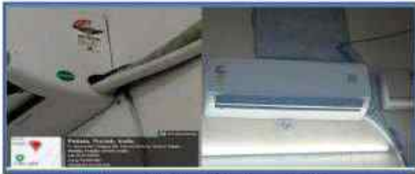
Energy Efficient Equipment: ACs
