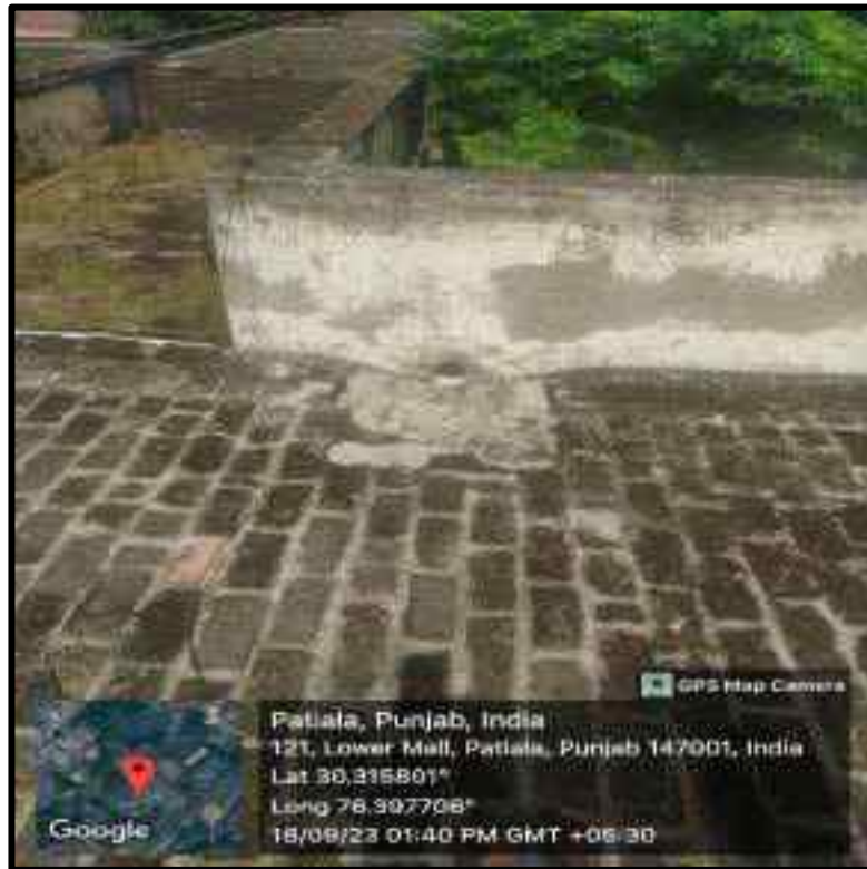
Collection pits having connecting from Rooftop to ground water through R.C.C. Pipes
