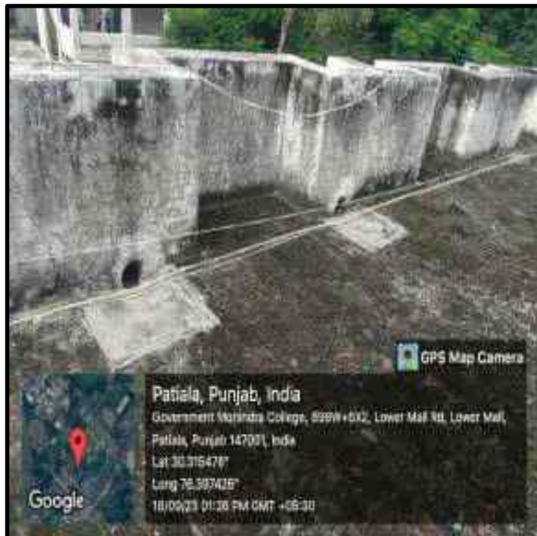
Collection pits having connecting from Rooftop to ground water through R.C.C. Pipes
