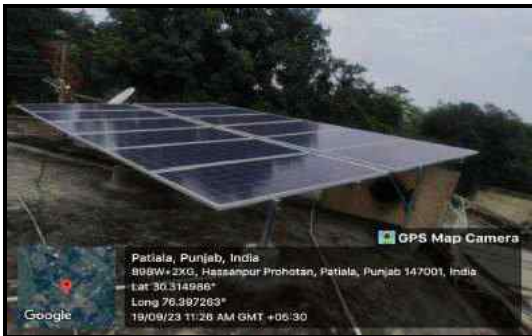
Solar Panel on the Main Administrative Building
