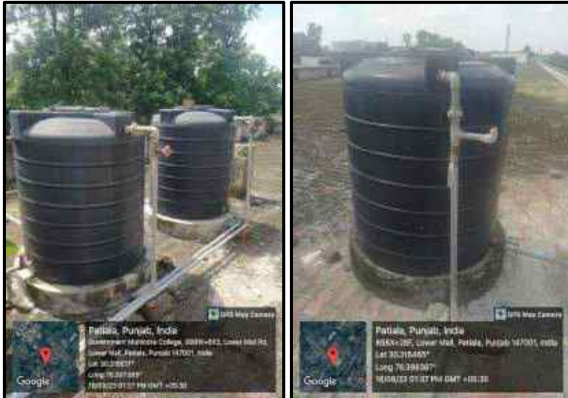
Water Storage Tanks
