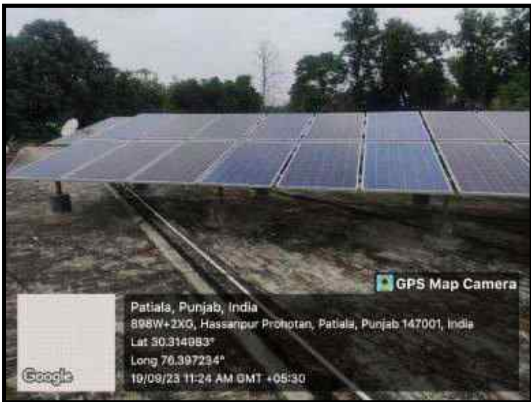
Solar Panel on the Main Administrative Building
