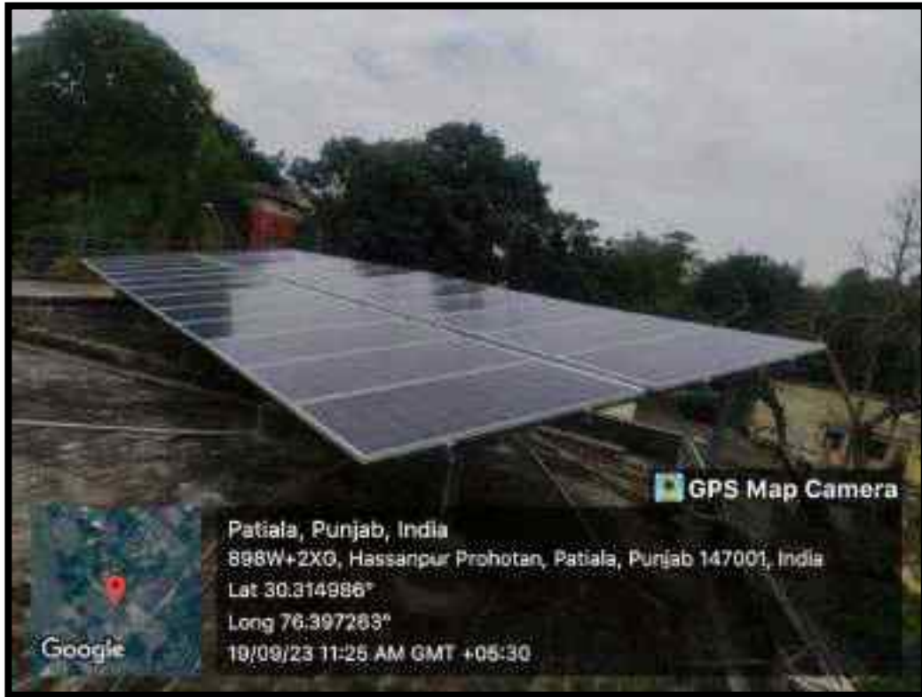
Solar Panel on the Main Administrative Building
