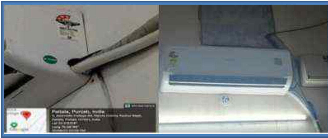
Energy Efficient Equipment: ACs
